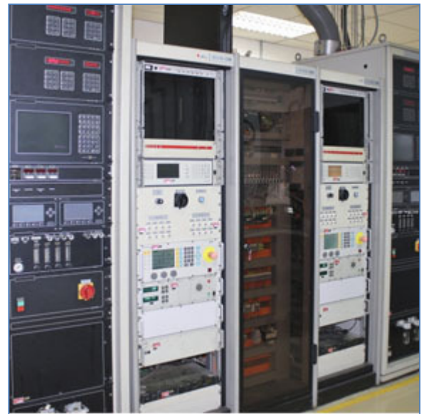
Equipment Room for Engine Dynamometer Laboratory at Delphi TCP.
