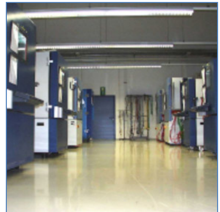
Thermal / Climatic Testing Chambers
